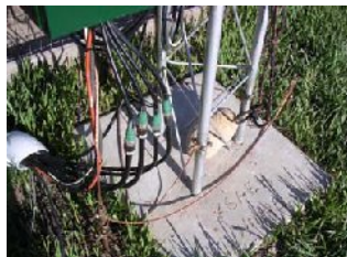
Tower grounding halo points
