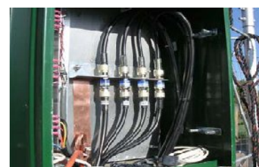
NEMA box with RF and DC Surge protectors
