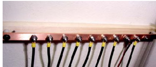
All radio equipment in the shack should be connected to a common ground copper buss bar. This bus bar is connected to the outside halo ground system via a short #2 GA copper ground cable.
