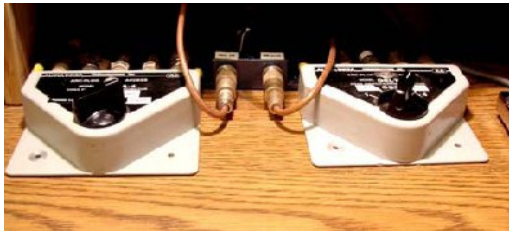
Use of a grounded antenna switch will aid in radio isolation during periods of non use, adding an extra layer of radio protection.
