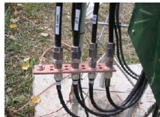
Tower base feed line ground connections.
